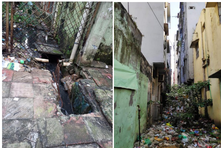
Figure 31 & 32 Shows:: Waste Water Drains & Gas Line
